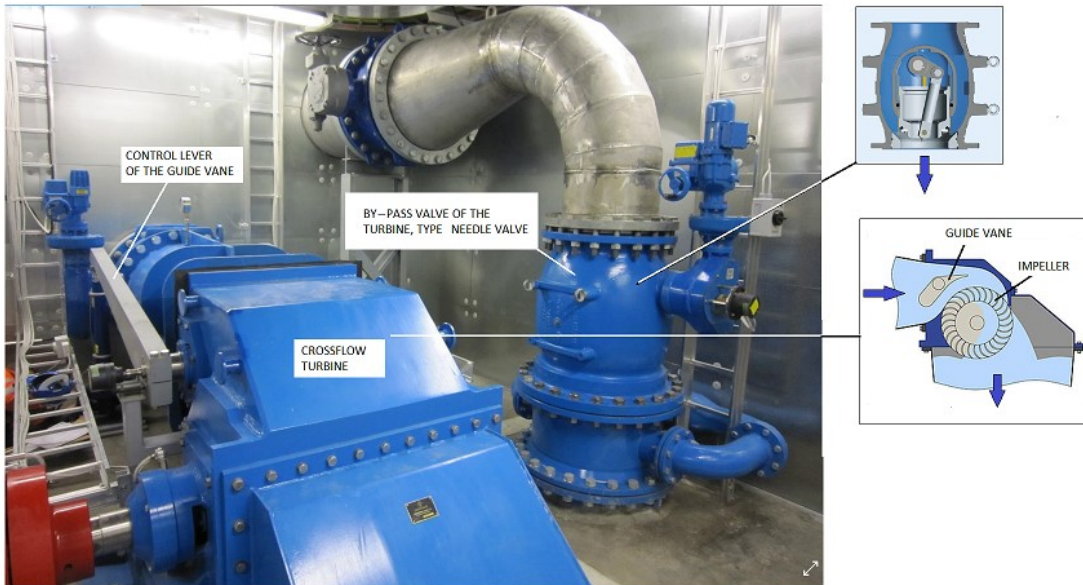
Figure 2.87 A Crossflow Turbine at the Discharge End of a Long Gravity Line.
